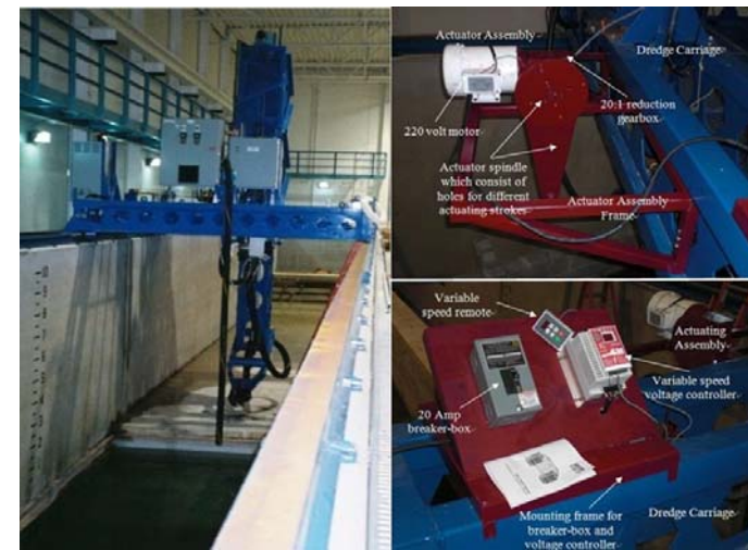
Fig. 2 Dredge/tow carriage (left), setup of actuator (upper right) and variable speed motor controls (lower right)
